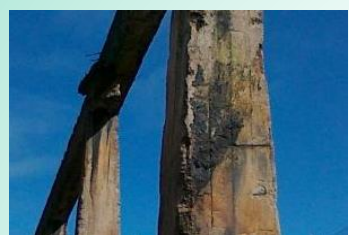
Carbonatation, corrosion chlorure
