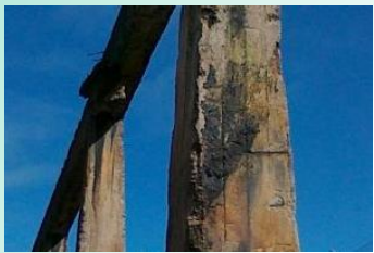
Carbonation, chlorides corrosion
